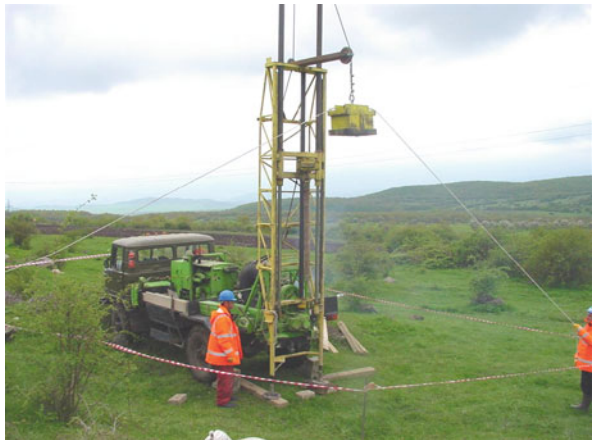
Fig. 1.19 Setup for a weight dropping trial used to measure peak particle velocities with distance
