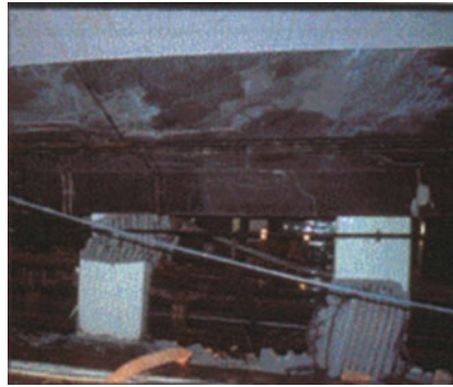
Fig. 11.11 Detail of collapsed columns of Daikai station (adapted from www.geerassociation.org/.../Kobe_1995/ch6-2.html )
