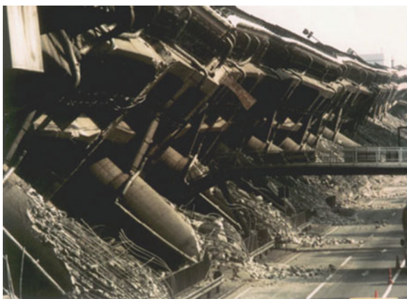
Fig. 10.16 A part of collapsed section of Hanshin Expressway in Japan (adapted from www.hp1039.jishin.go.jp/eqchreng/f7-15.htm )
