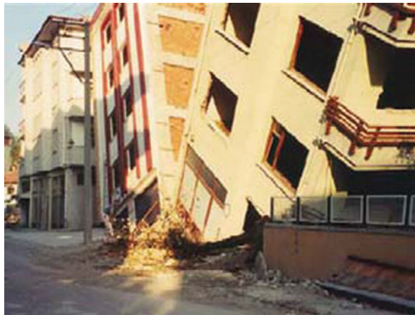
Fig. 9.10 Terveler (on the right side) and the adjacent building tilt in Adapazari – Turkey (adapted from http://www.nibs.org/client/assets/files/bssc/Topic15-4-GeotechnicalEarthquakeEngineeringNotes.pdf )
