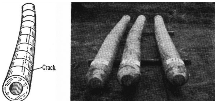
Fig. 10.15 Cracked pre-cast reinforced concrete piles from Yachiyo Bridge during the 1964 Niigata earthquake in Japan (Meymand, 1998)
