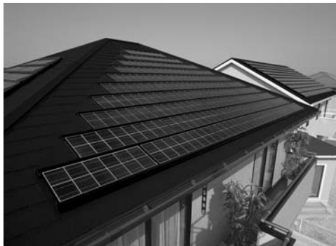
Fig. 6-3: Solar cells installed on a roof of a house (Courtesy of KYOCERA Solar Corporation)
