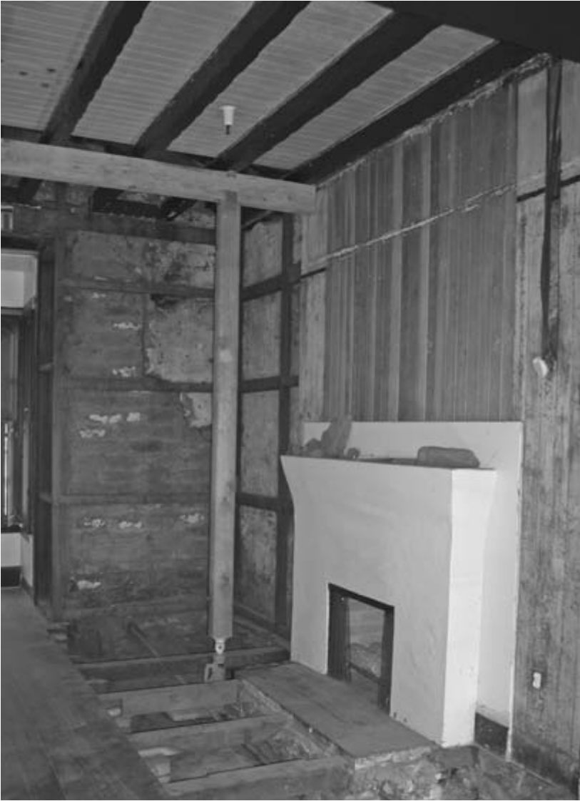
FIGURE 11. Interior excavation of the Officers' Club to expose Spanish-colonial adobe walls and packed clay floors.
