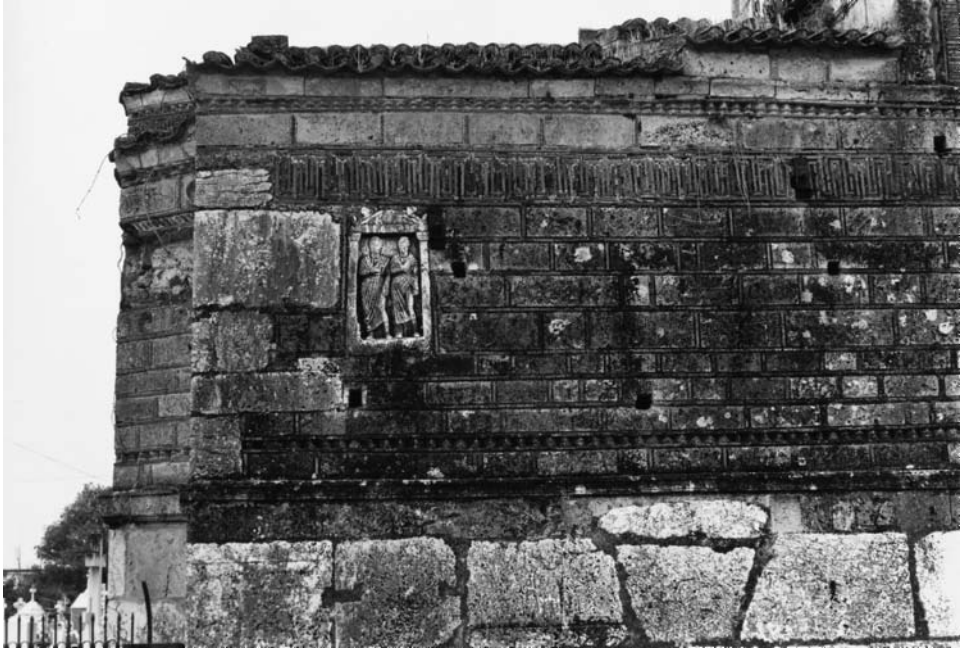
Plate 4.2 Church of the Virgin at Merbaka. Detail of north facade (photo by the author)
