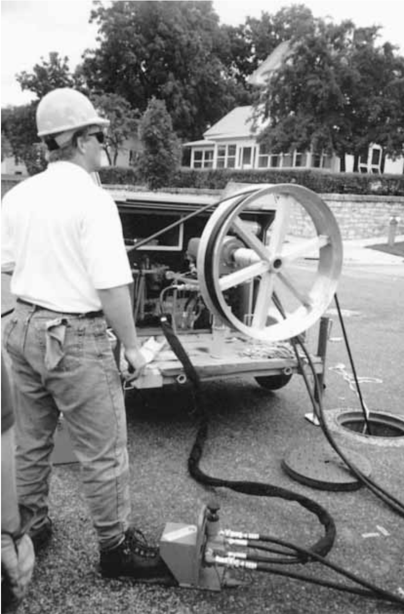
Figure 4-8 For long pulls, the mechanical puller applies consistent tension and monitors it to prevent overstressing the fiber.
