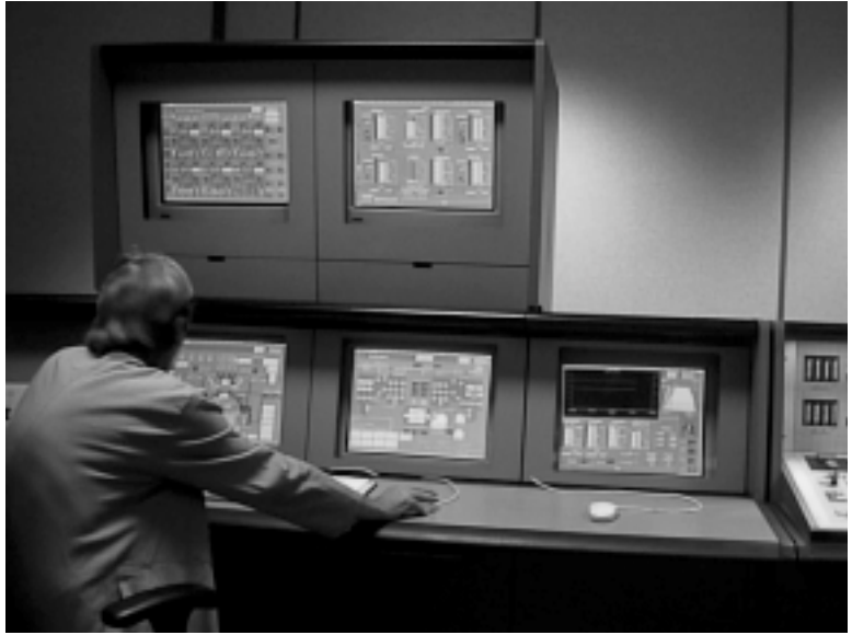
Figure 1.6 Using a mouse to control a power station. The state-of-the-art control room at Ironbridge Power Station, Shropshire, uses computer monitors to display data readings taken at dozens of points in the steam-producing plant, in the turbines and in the electricity generators. The operator controls the power station by calling up a virtual control panel on the monitor. On this, the usual control switches, variable resistors, indicator lamps and meters are displayed in diagrammatic form. There is no keyboard on the computer. Instead, the operator uses a mouse to operate the controls, clicking on 'buttons' or dragging 'sliders' in just the same way as when playing a computer game. The station also has a basic conventional control panel with real switches for back-up in case of computer failure. (By courtesy of Eastern Generation Ltd.)
