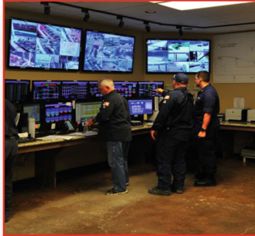
Fig. 6.2 Coast Guard personnel observing the security and safety control systems at a marine terminal. USCG photo
