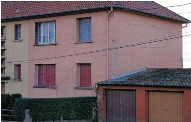
Fig. 33. Damaged house because of surface subsidence above an abandoned iron ore mine in Roncourt, Lorraine/France.
