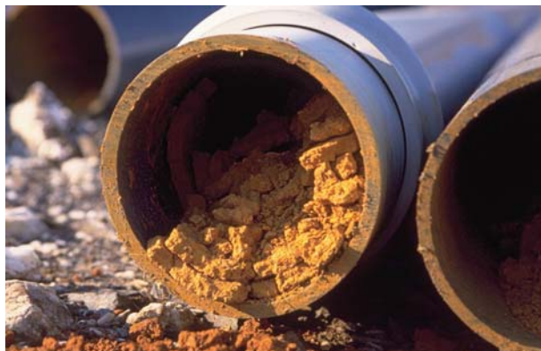
Fig. 8. Ochre precipitates in a mine water discharge pipe of the abandoned Straßberg/Harz fluorspar mine.
