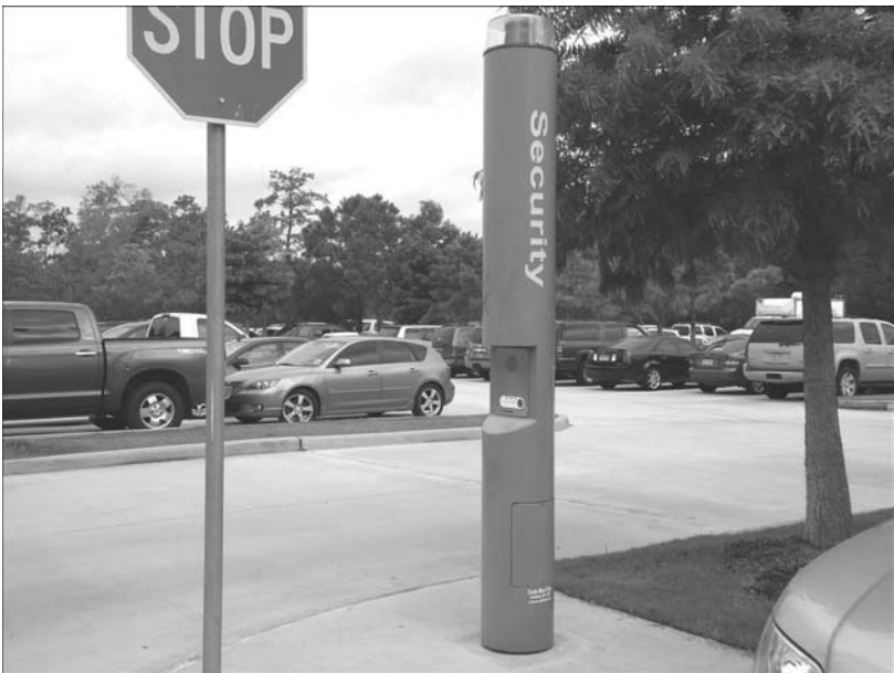
FIGURE 10.6 Exterior emergency telephone/speaker/light tower.
