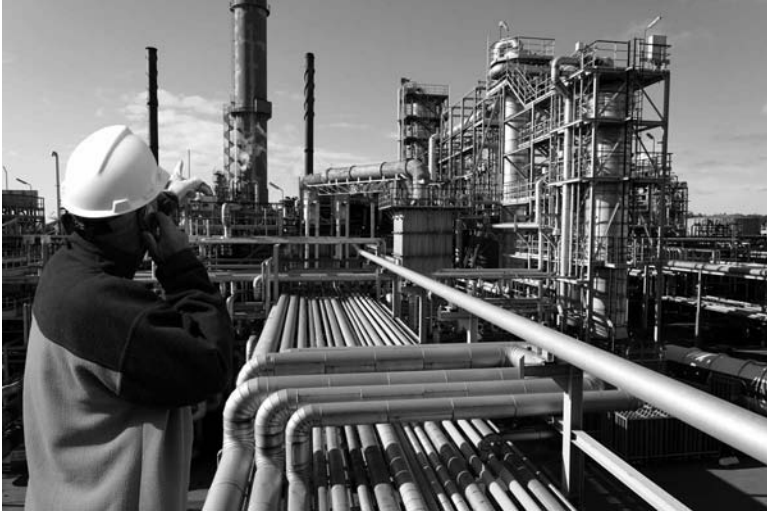
FIGURE 5.3 Oil and gas refinery pipelines. (Courtesy of Shutterstock.com.)
