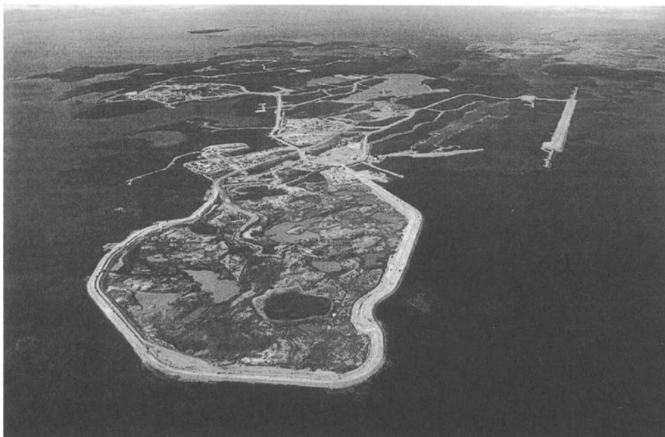
FIG. 6 Project site in 2002 showing construction of dikes to keep lake water from the mining pits
