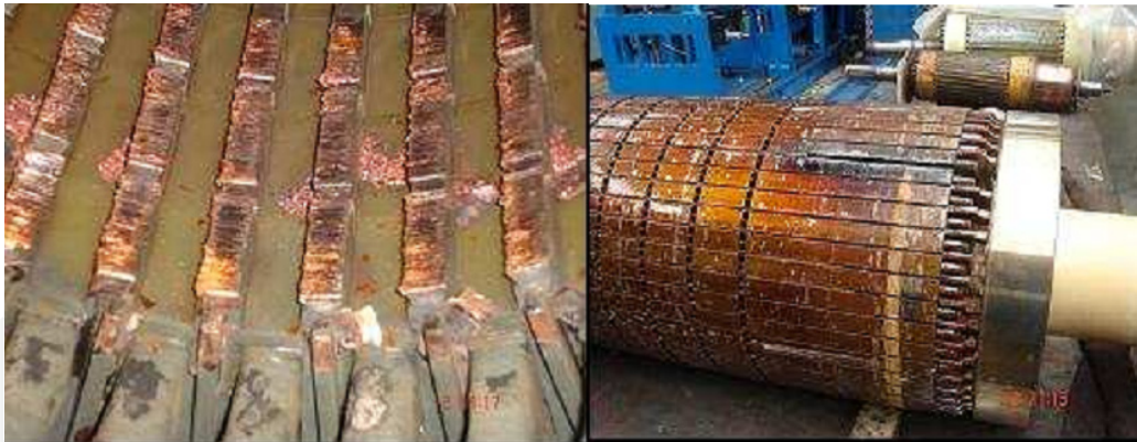
Figure 26. Stator and Rotor Damages
