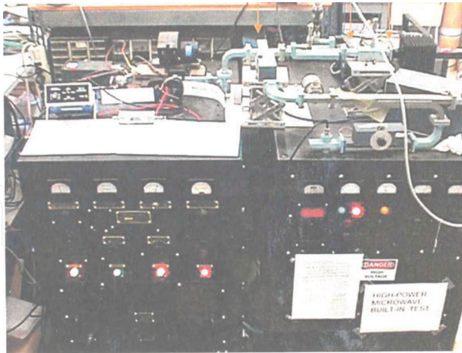
Figure 5.8. Magnetron (center) with waveguide (right) on the top of power supply and pulser cabinets.
