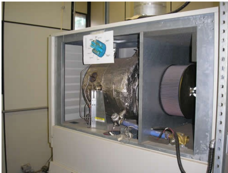
Figure 7. Capstone microturbine in the laboratory at UNIFEI.
