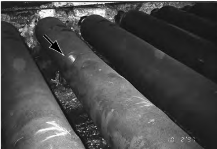
FIGURE 5.8 Blistering of conventional furnace roll.
