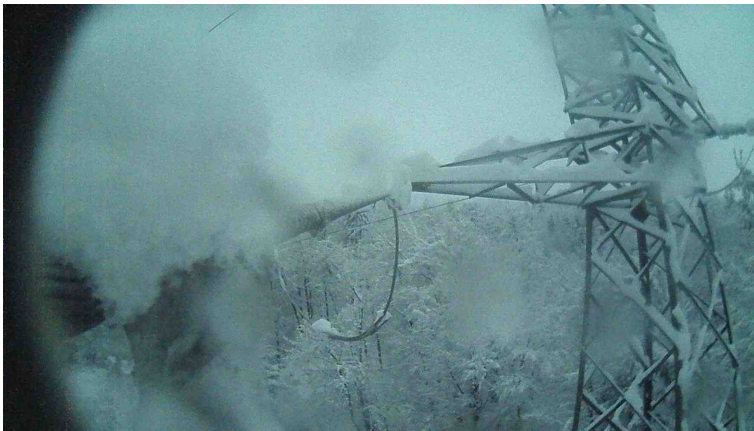
Fig. 6. Real state of a phase conductor - 18 January 2019
