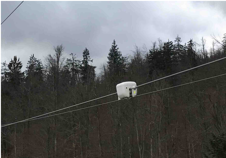
Fig. 1. OTLM line monitoring sensor
