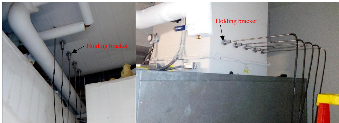
Figure 2-9: Hot-wire velocity probe mounting in AHU-6 for performing traverse measurements.
