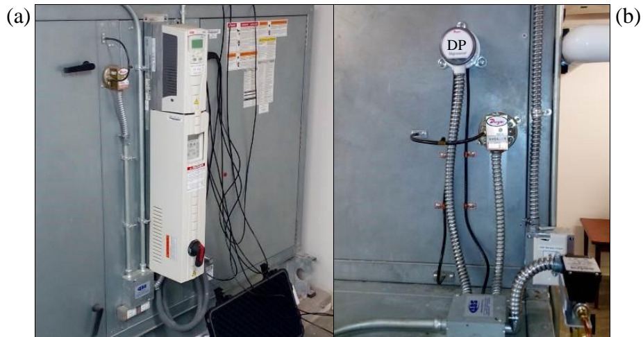
Figure 2-6: VFD for RF and DP sensor installed across the SF.
