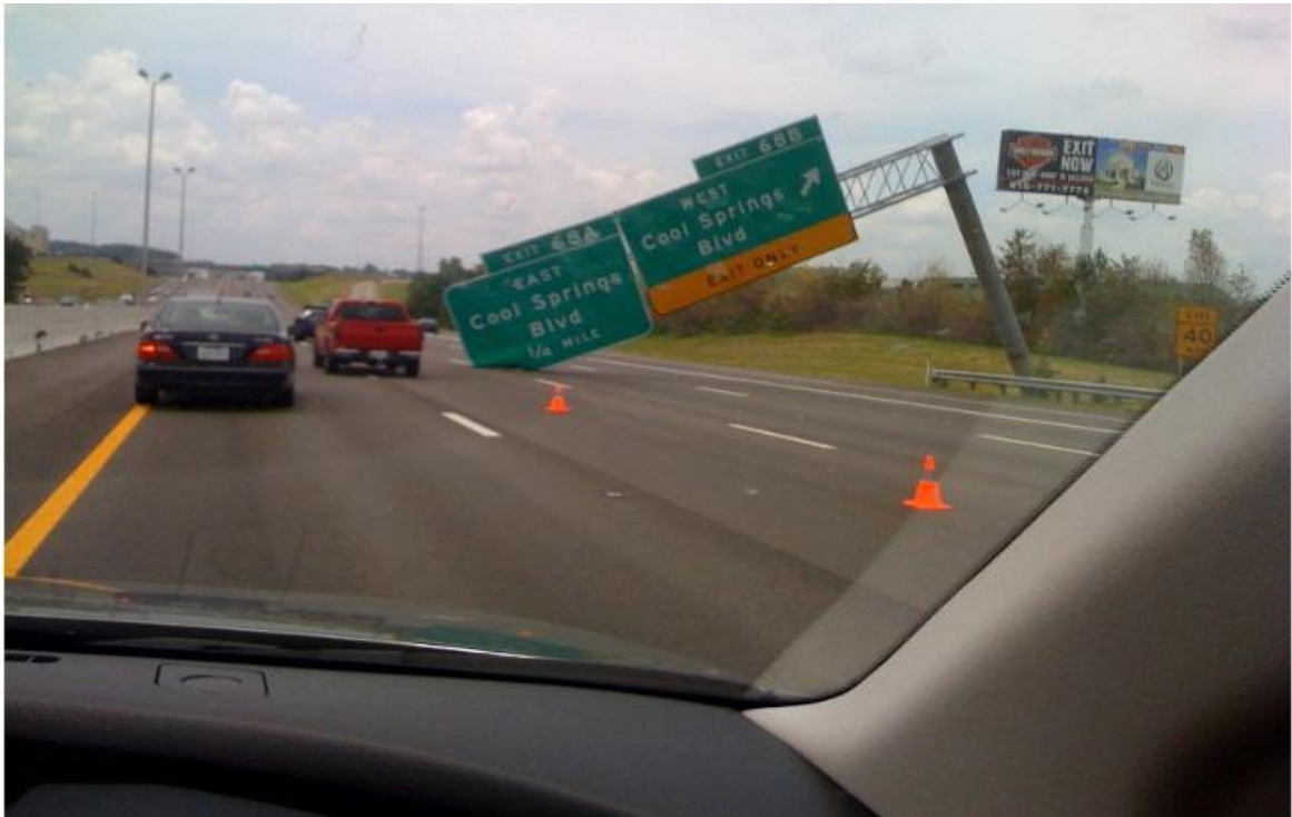
Figure 1-2: Failure of cantilever sign support structure along I-65 in Tennessee
