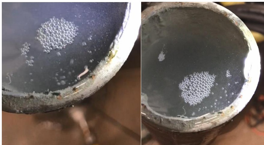
Figure 62: Fly ash cement showing leak position (Small Setup 1 Experiment 6).
