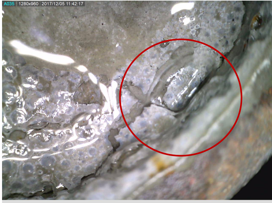
Figure 65: Cement after leak
