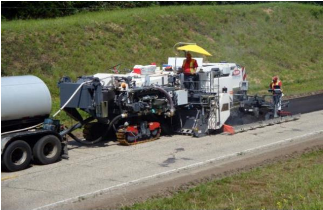
FIGURE 1 Single Unit Recycling Train (7)
