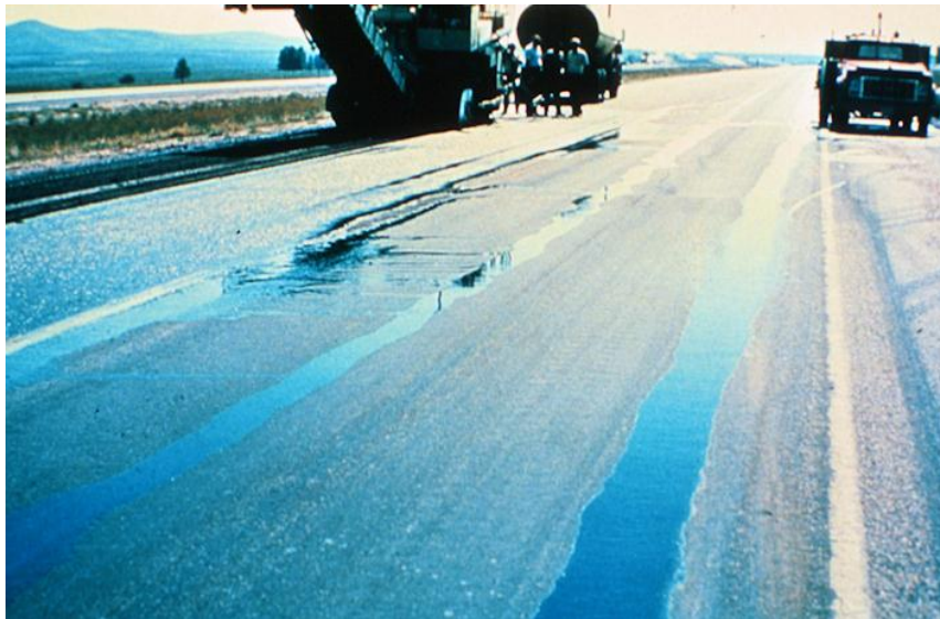
Figure 2.15 Pavement rutting track
